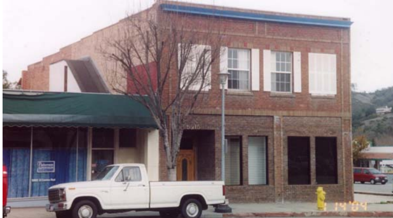
Figure 2. Retrofitted unreinforced masonry buildings such as this one in Atascadero generally performed better than nearby unretrofitted or partially retrofitted buildings. (Photo: CSSC)
